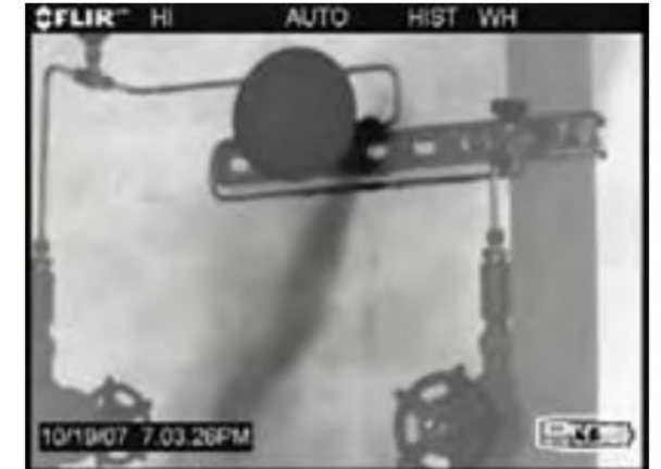
A leaking pressure gauge
